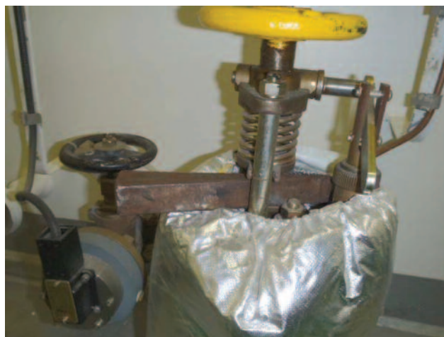
Quick closing valve held open with a steel wedge
