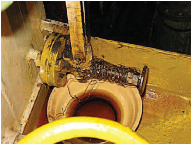
Self-closing gauge glass valve gagged with wire
