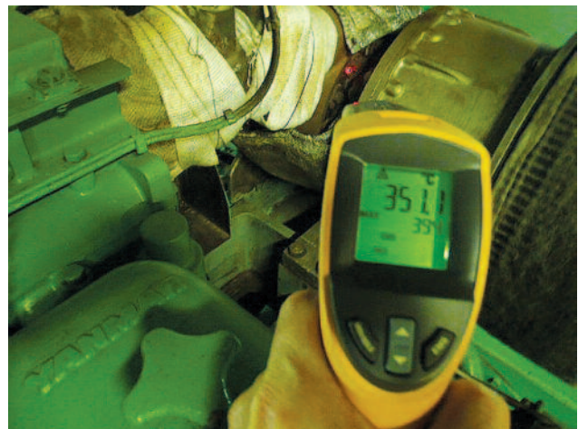
"Hot spot" due to missing insulation
