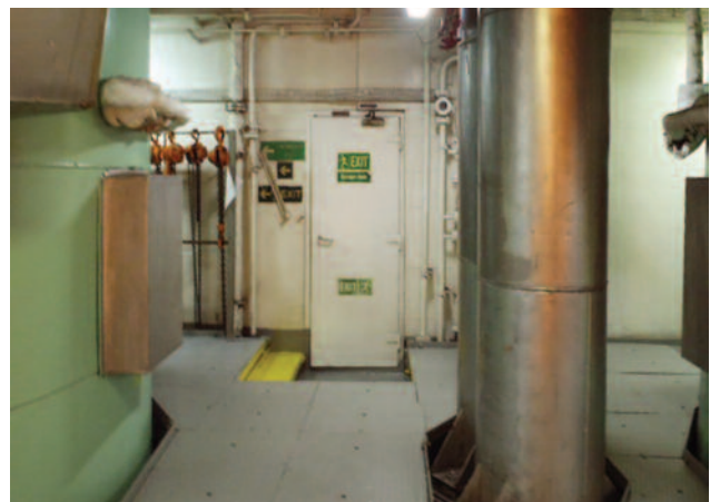
Poorly marked escape route and door
