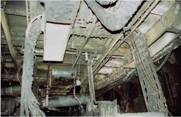
Fire spread along cable trays away from an auxiliary generator where the fire originated
