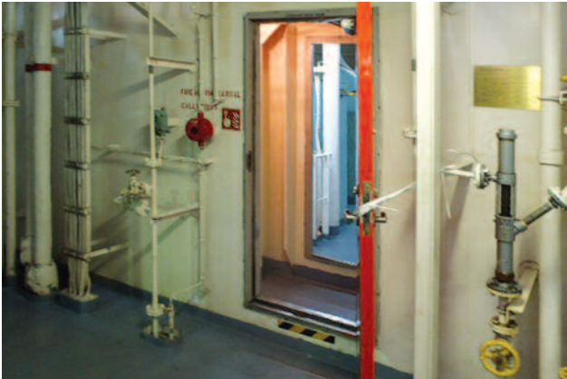
Steering gear fire doors tied open
