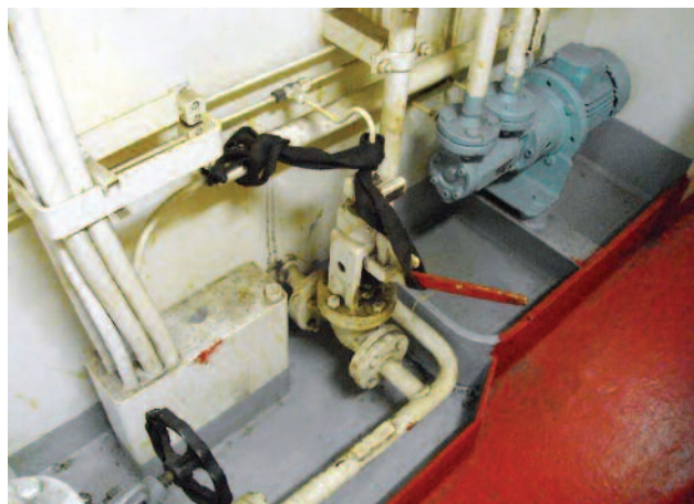
Quick closing valve held open with a strop
