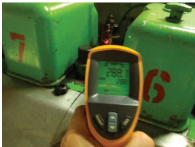
Uncovered indicator cock with exposed temperature above SOLAS limit
