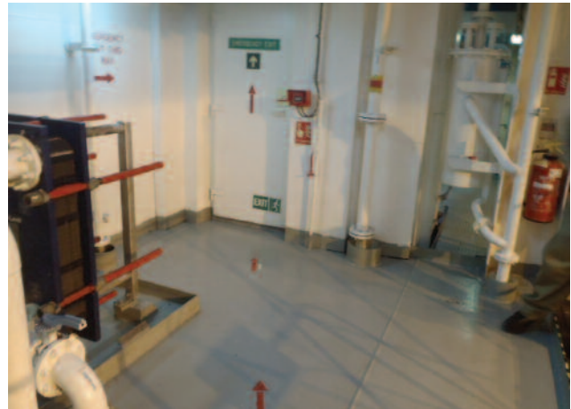
Well marked escape route arrows
